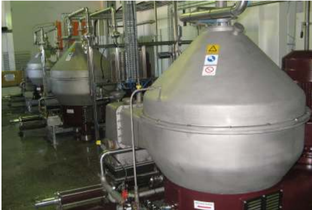
An STS Series Clarifier installation at a South African beverages plant
